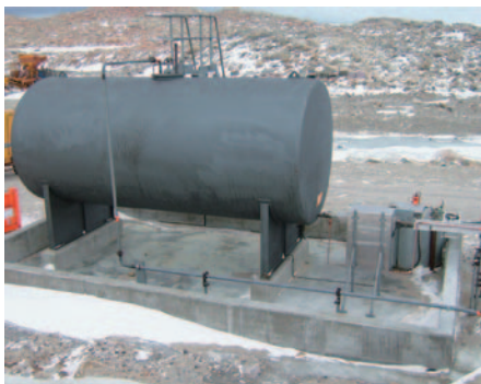
Photo 17 燃料タンクとコンクリート防油堤 Photo 17 A fuel tank enclosed by an oil retaining wall.
