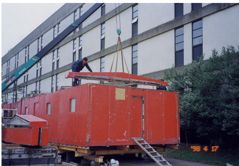
図9 居住棟の復元工事3 屋根パネルの設置 Fig. 9. Reconstruction of the living hut. Third phase: Installation of roof panels.
