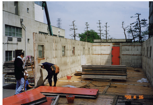
図8 居住棟の復元工事2 壁パネル建て込み Fig. 8. Reconstruction of the living hut. Second phase: Assembling of wall panels.
