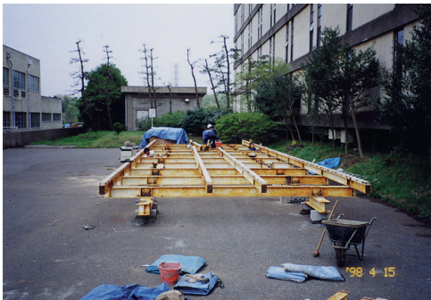
図7 居住棟の復元工事1 大梁, 小梁, 根太の組立 Fig. 7. Reconstruction of the living hut. First phase: Steel work.
