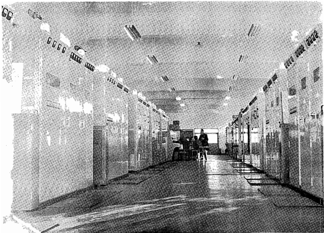
写真8 銚子無線局の送信機室(何れも TV 1301 型送信機) Photo. 8. 3 kW transmitters at Choshi Radio Station.
